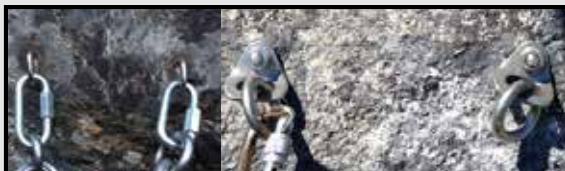
Two versions of recent anchor replacements, glue in bolts and quick-links (left) and mechanical bolts with rings (right)
